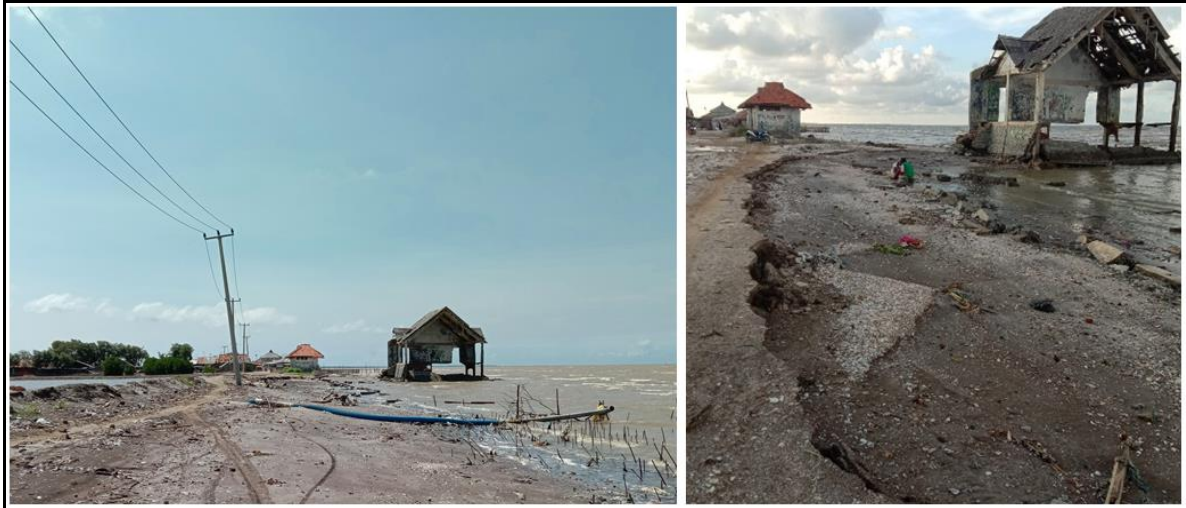
Figure 2. Damage to the beach and tourist facilities due to coastal erosion at Cilamaya Kulon Beach area.
